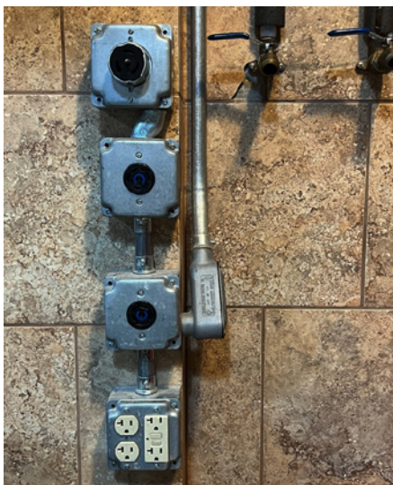
Electric receptacles at the Blichmann brew lab.
