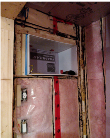
During construction an opening was created for a through-wall air conditioner to cool the room.
