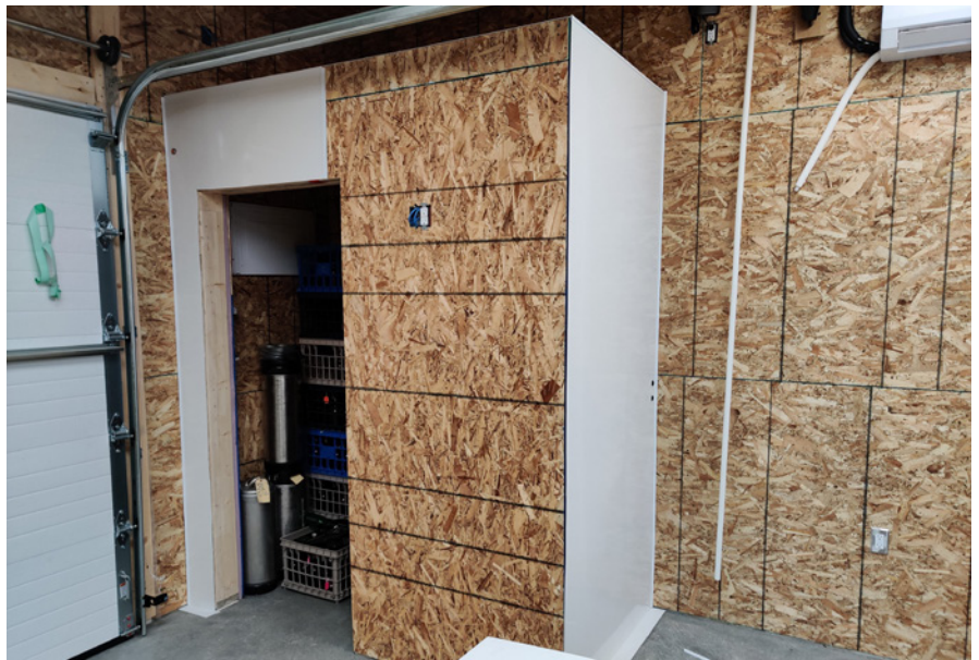
A fiberglass-reinforced plastic gives a finished look to the wall over oriented strand board for strength.
