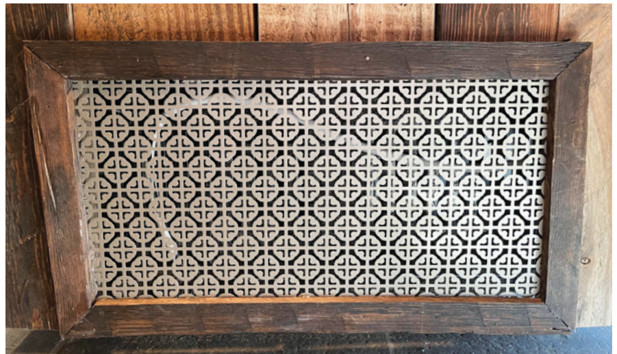
In order to give the chest freezer ample ventilation to dissipate heat, an old-timey metal grate was used to create the necessary air flow. Lack of ventilation can kill the compressor if not properly addressed.
