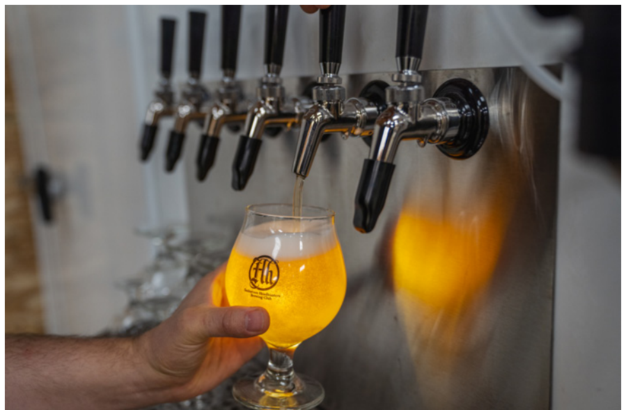
The completed six-faucet draft system from the outside of the cold room.
