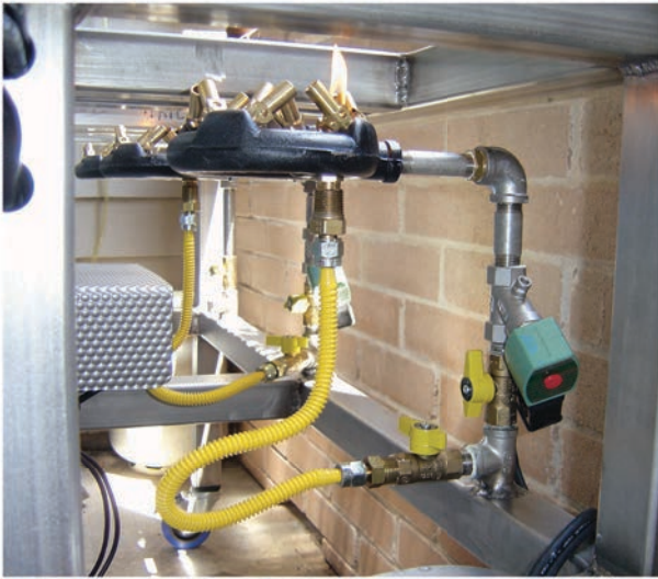
A close up of one of the burners and associated plumbing. The flexible yellow line leads to the pilot light for that burner. The hard piping is opened and closed by the ASCO switch. See page 6 for a diagram of the assembly.
