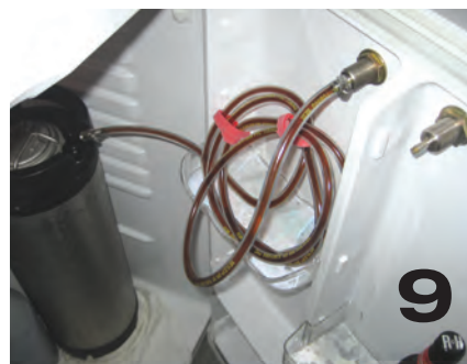
Beverage line connects the "beer out" post to the tap on the kegerator. Keeping these lines clean is very important.
